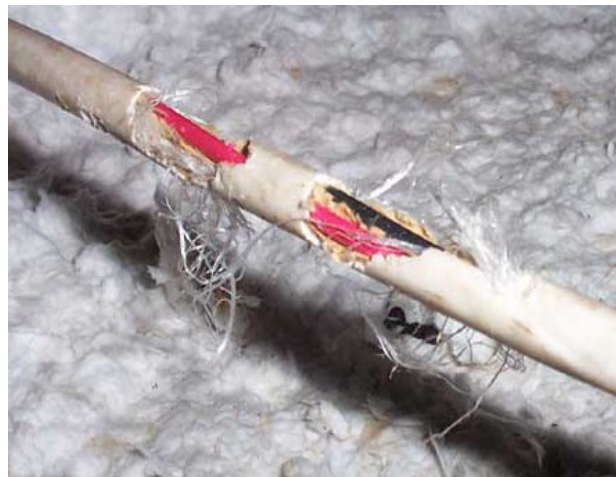
This shows the type of damage a squirrel causes to wiring.
