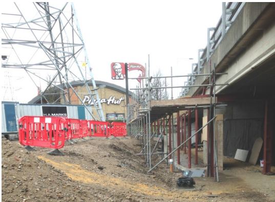
The South Wall has now been demolished to be replaced with a glass and a new entrance.
