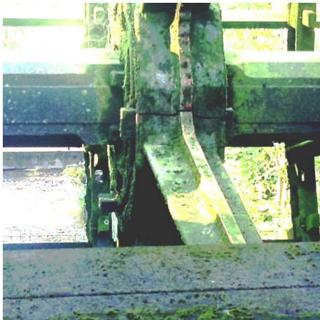
The crack appears.
