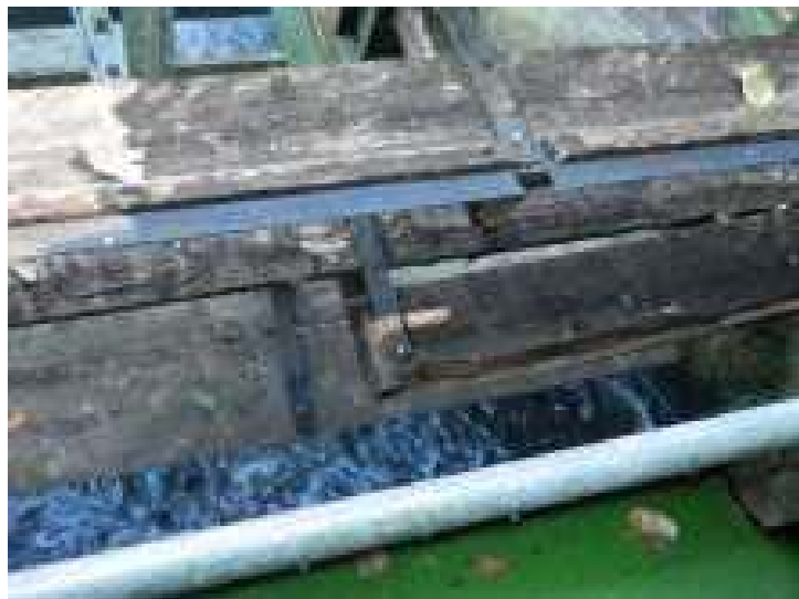
Figure 8 - Illustrating the urgent need for refurbishment of the water wheel
